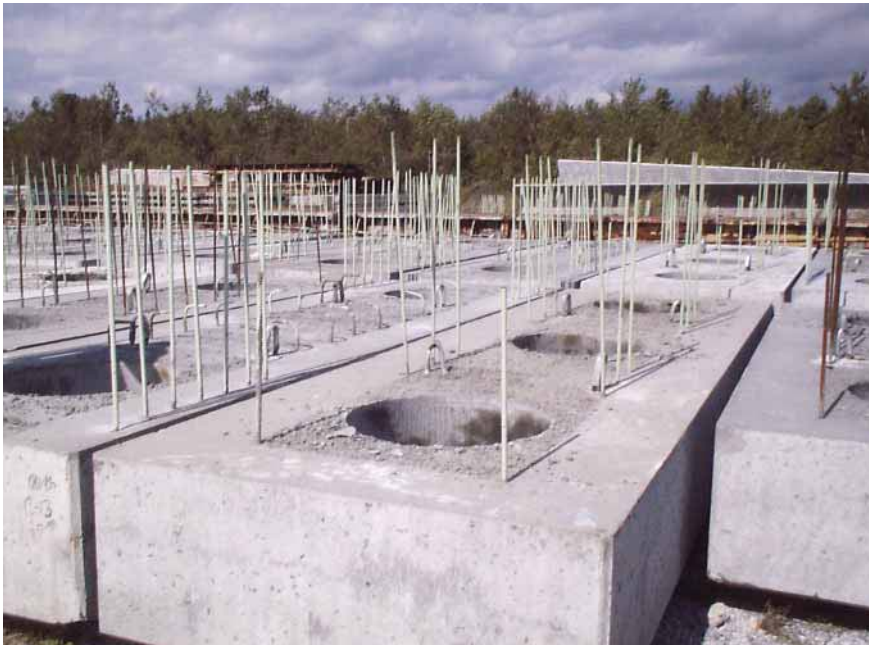
Fig. 9. Precast pile subcaps in staging yard. Careful detailing of subcaps translated into a smooth integration and connection with deck and pile elements. Photo courtesy: Guy F. Atkinson Construction Company.
