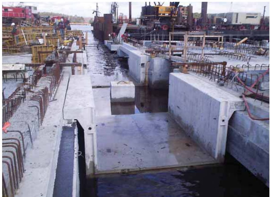
Fig. 11. At high tide, precast transverse beam detailing provides support for both the utility vault and deck panel/vault lid while hanging clear of the pile caps below. Photo courtesy: Guy F. Atkinson Construction Company.
