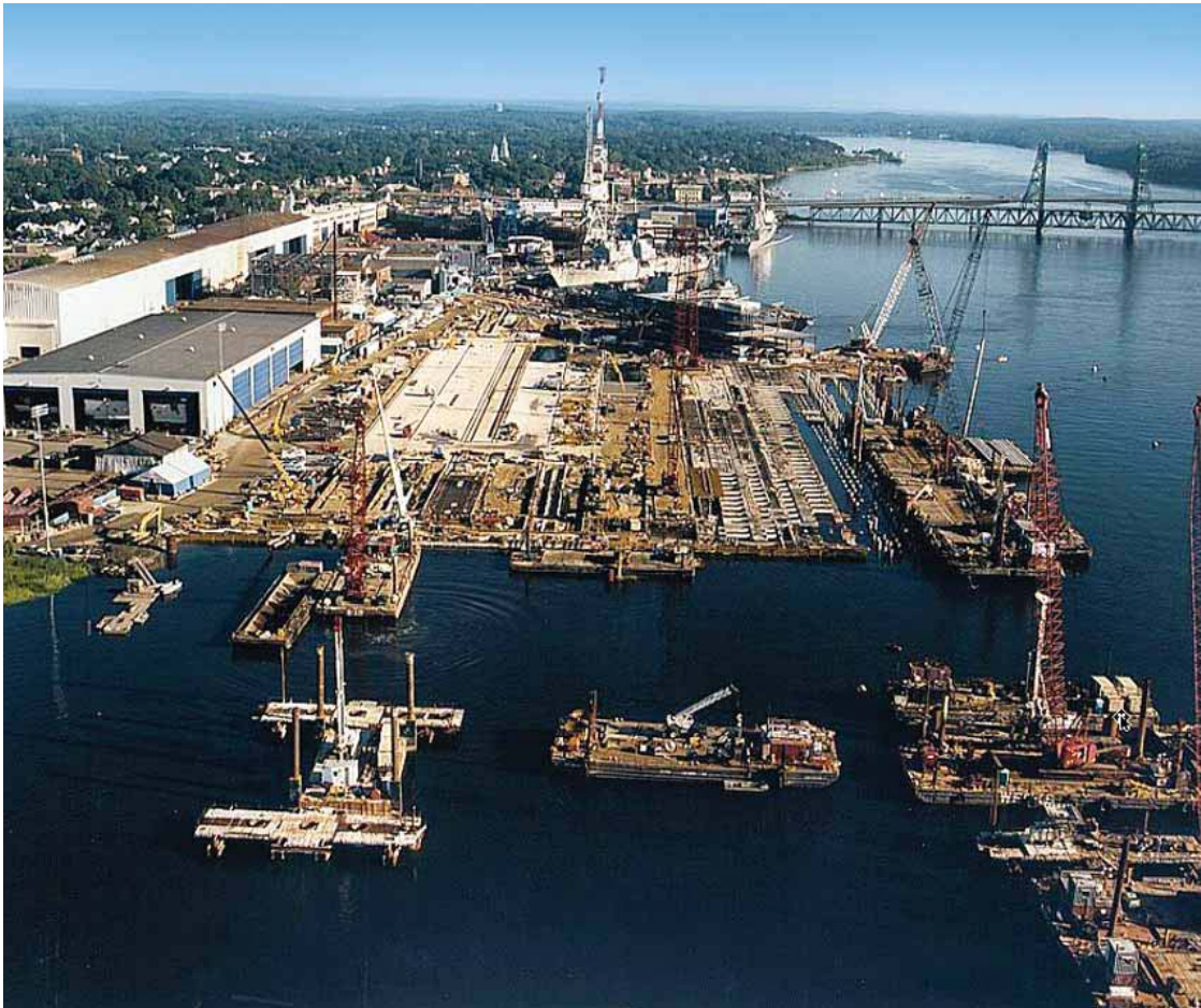
Fig. 19. Overview of project showing numerous barge-mounted cranes operating at the Bath Iron Works construction site.
