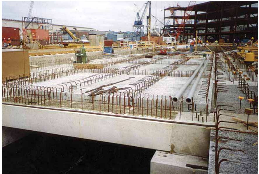
Fig. 14. The precast deck panel was limited to an 8 in. (203 mm) depth, too thin for shear key performance. Special nonlinear finite element analysis demonstrated that the composite topping was sufficiently stiff for adequate load transfer. Photo courtesy: Guy F. Atkinson Construction Company.
