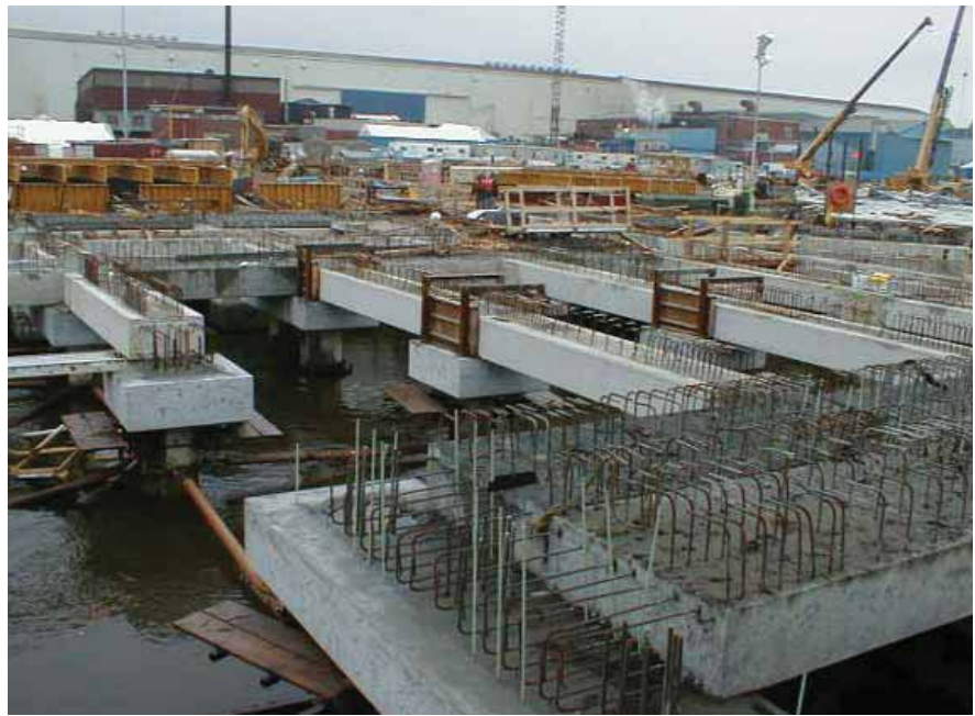
Fig. 10. Precast design flexibility meant that the deeper longitudinal craneway beams and transverse beams could be erected at the same elevation. Note that four precast members rest on a single pile cap without interference to numerous reinforcing elements. Photo courtesy: Guy F. Atkinson Construction Company.
