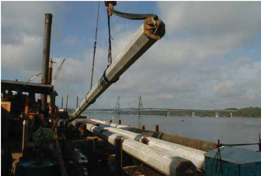
Fig. 12. Precast piles being lofted with specialized rigging. High strength concrete was used in the 28 in. (710 mm) solid octagonal section piles with spiral reinforcement to provide both strength and ductility. Photo courtesy: Guy F. Atkinson Construction Company.
