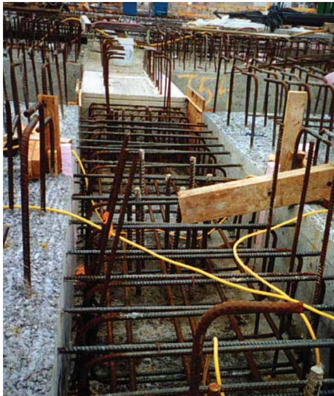
Fig. 17. Careful coordination was required to ensure that bars projecting from piles, subcap, transverse beams and longitudinal beams did not create interferences during erection. Photo courtesy: Guy F. Atkinson Construction Company.
