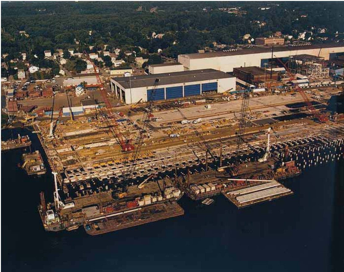
Fig. 18. Aerial view (looking west) shows construction sequence at the Land Level Transfer Facility. The total project added 15 acres (6 ha) of the modern shipbuilding facilities in Bath, Maine. Photo courtesy: Bath Iron Works.
