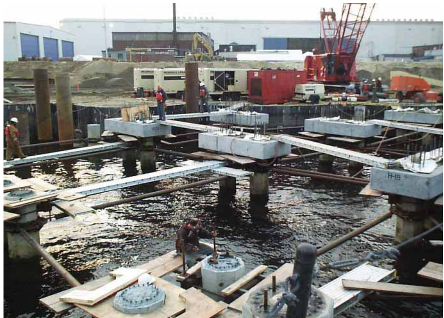
Fig. 15. Once the precast piles were driven to refusal in the pre-drilled rock sockets, temporary bracing was installed to maintain position until the final deck integration. Photo courtesy: Guy F. Atkinson Construction Company.
