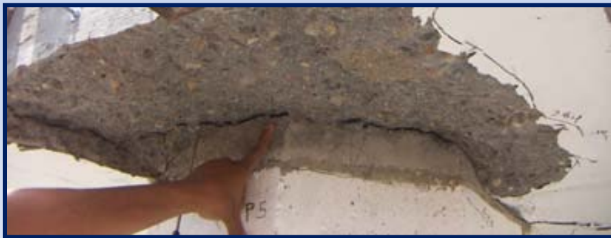
Deck Prying Spall & Interface Gap
