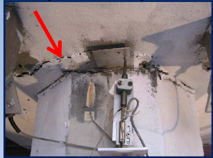
Deck Crushing \mu_{\Delta} = 2 (1.6% drift)
