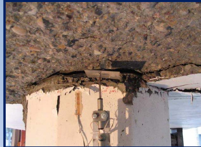
Spall Removed \mu_{\Delta} = 4 (2.3% drift)
