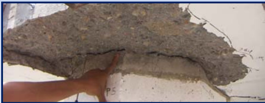
Deck Prying Spall & Interface Gap
